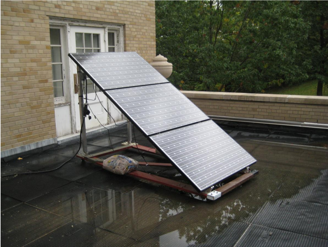
Figure 7: The Photovoltaic Display .
